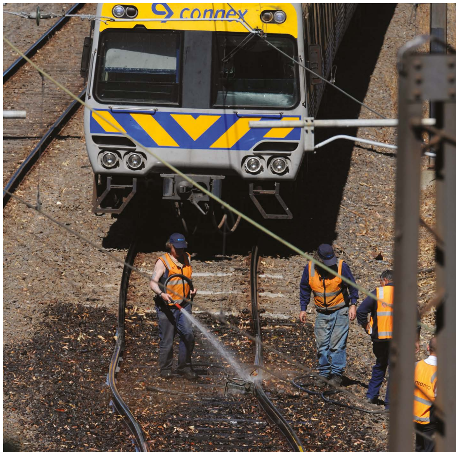
Cooling railway tracks with water or by using white paint can reduce rail buckling.
